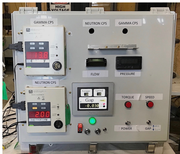
Sample of a Remote Control Station
